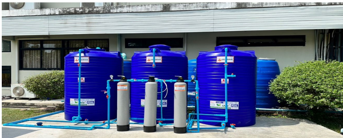
A system of rainwater filters
