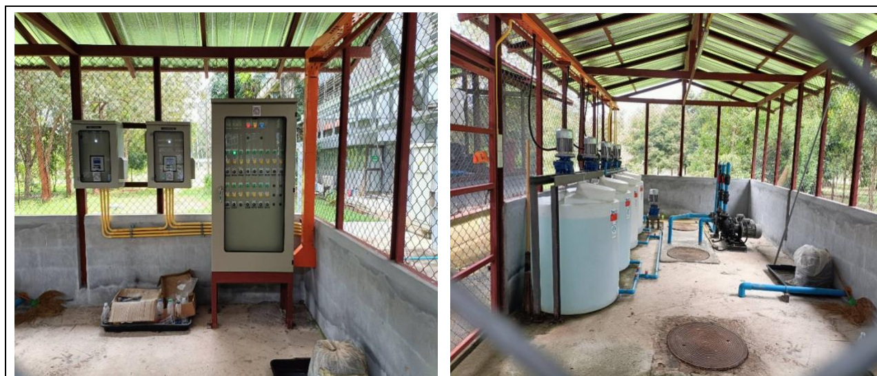
Sewage Disposal (Suratthani Rajabhat University, Thailand)
