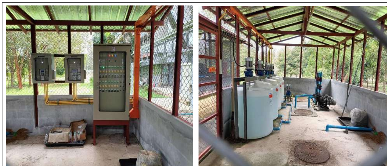
Sewage Disposal (Suratthani Rajabhat University, Thailand)
