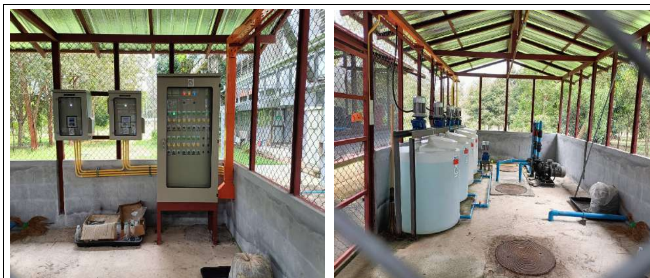
Sewage Disposal (Suratthani Rajabhat University, Thailand)
