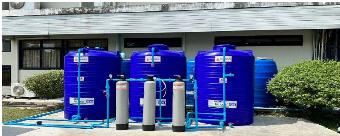
A system of rainwater filters
