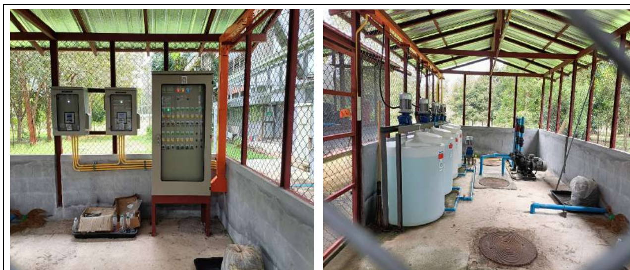
Sewage Disposal (Suratthani Rajabhat University, Thailand)
