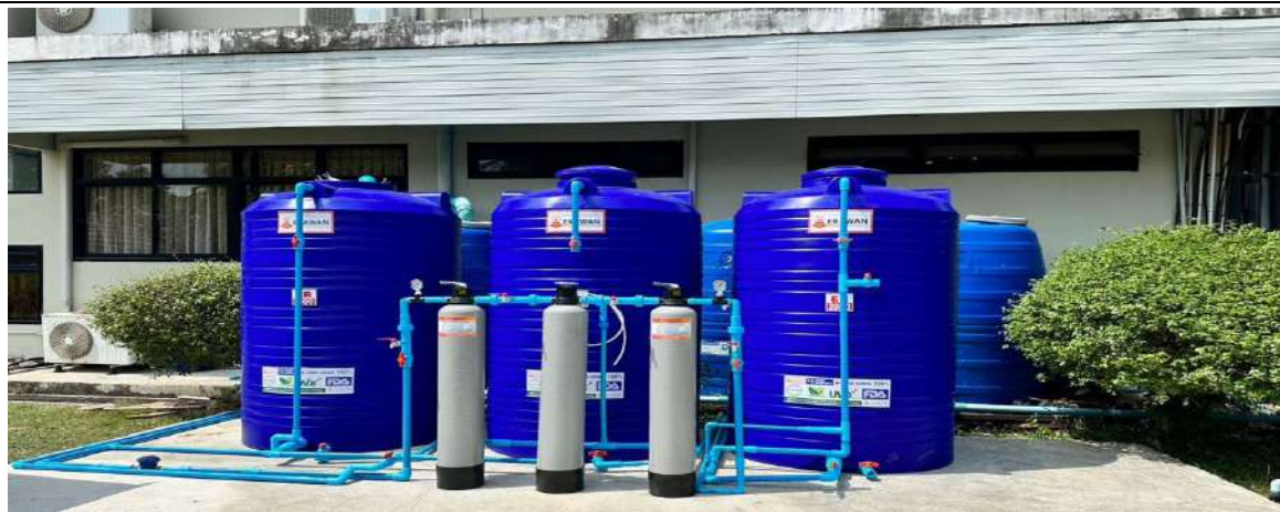
A system of rainwater filters
